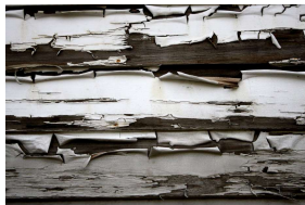
Damaged Legacy Lead Paint
